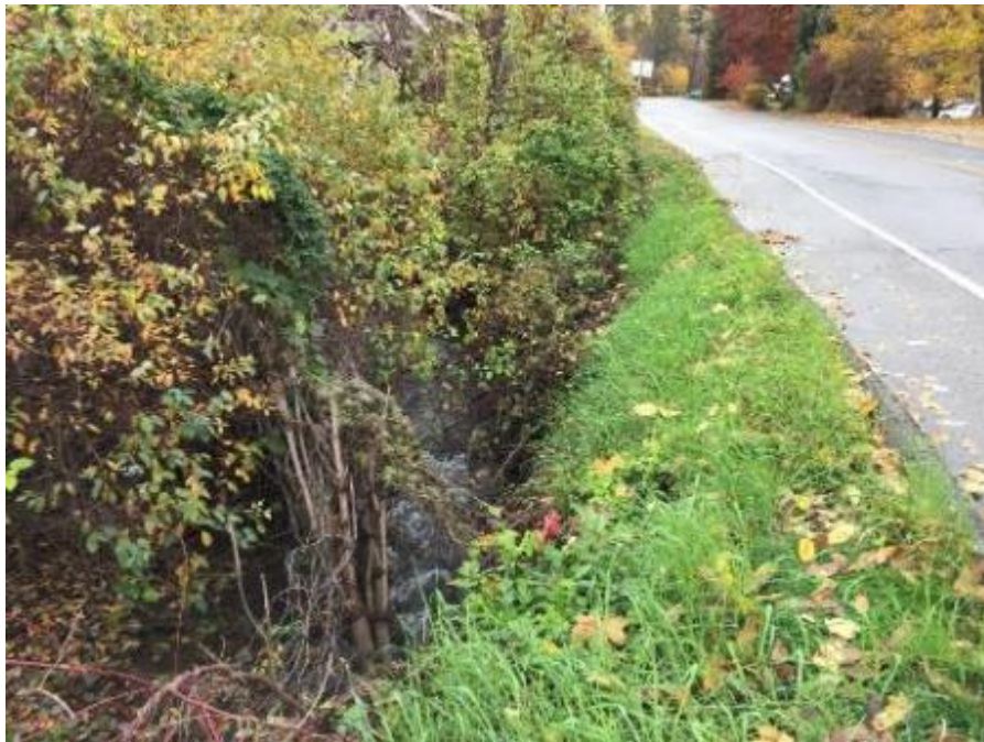
Figure – Bank Erosion near Road Embankment
