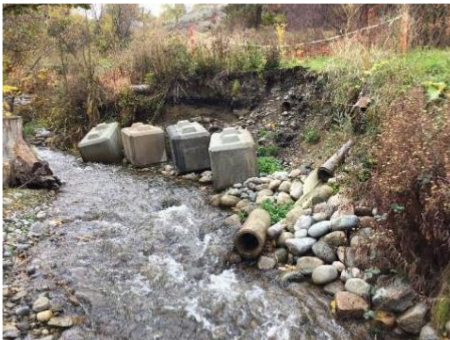
Figure – Lock Blocks and Bank Erosion
