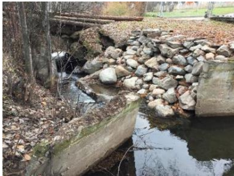
Figure – Creek Obstruction
