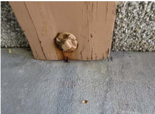
Photo S3 Column base at entrance with termite damage below bolted connection. Repair is recommended.
