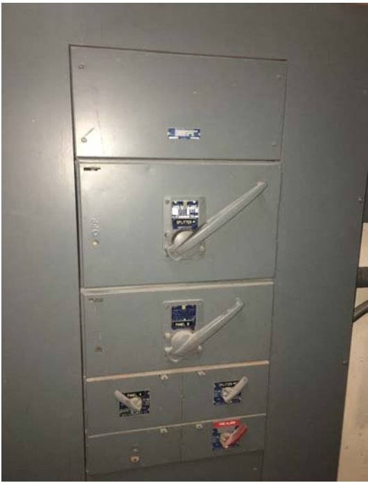
Photo E1 Section of Main Switchboard
