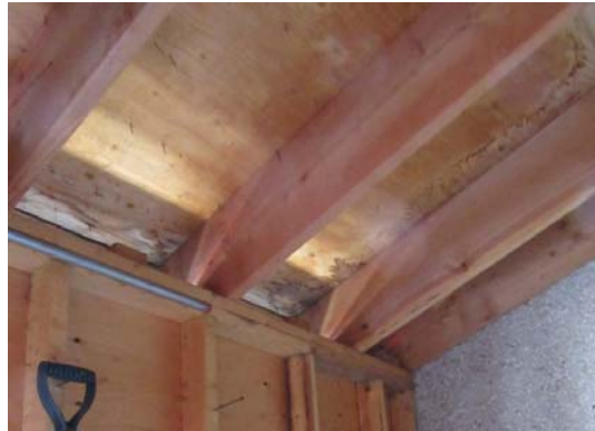
Photo S10 Plywood roof sheathing is in bad condition.
