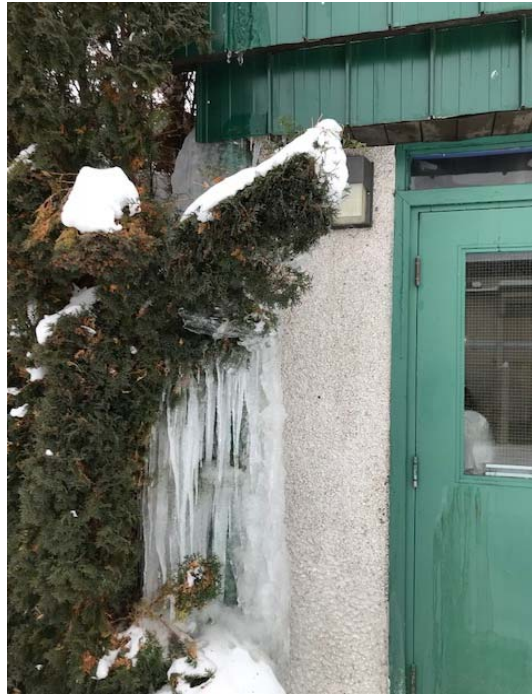
Photo Client6 View of ice buildup typical at downspouts.
