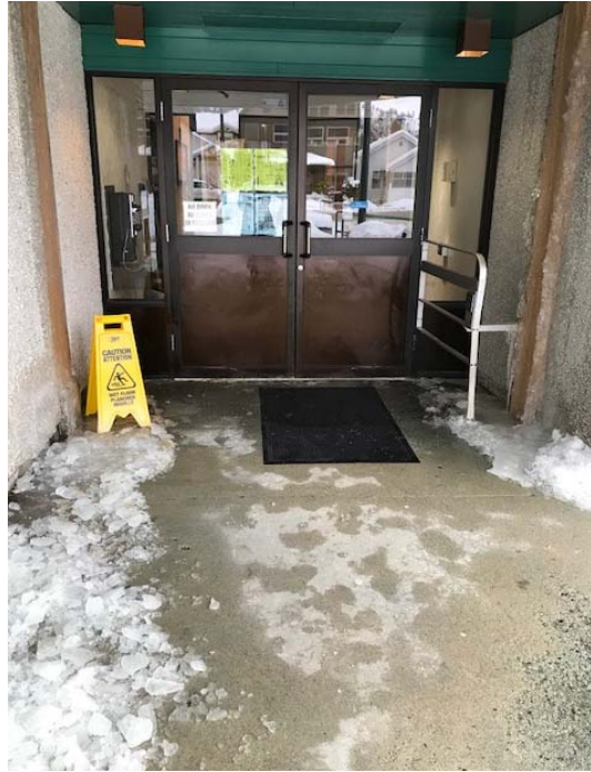
Photo Client2 View of main entrance during winter with ice.
