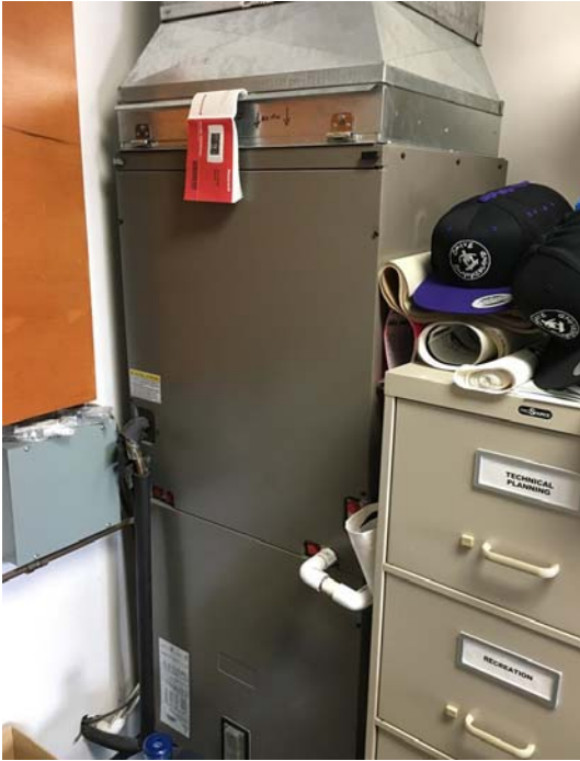
Photo M2A Office Space Heat Pump Unit
