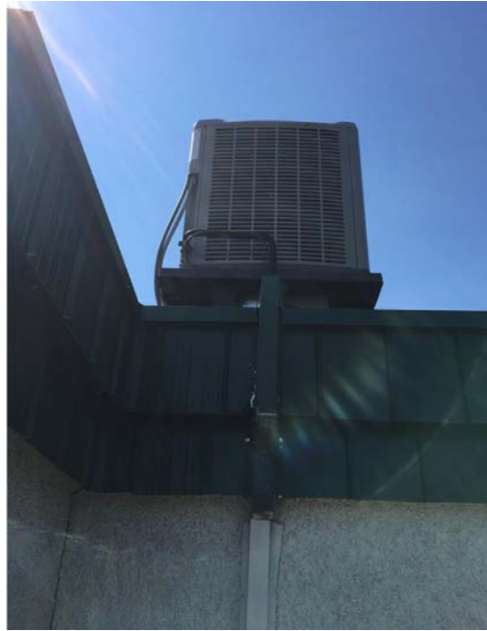
Photo M2B Office Space Condenser Unit
