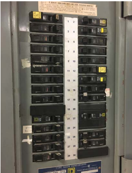
Photo E4 Panel SB Breakers
