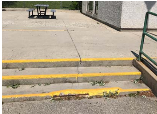
Photo S6 Deteriorated stair nosing
