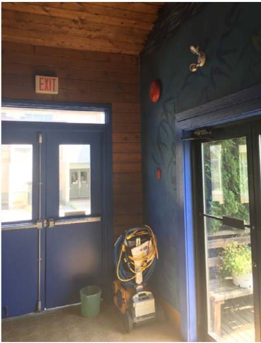
Photo E8 Exit Emergency Light / FA Bell /FA Pull station
