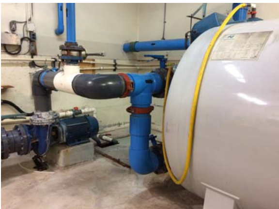
Photo PSys1 Main Pool Piping
