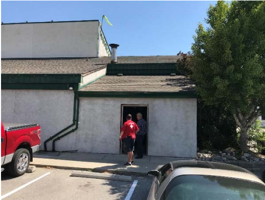
Photo A7 View of storage room added to exterior of the building.
