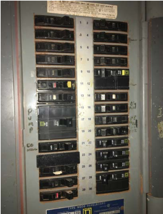
Photo E2 Panel A Breakers
