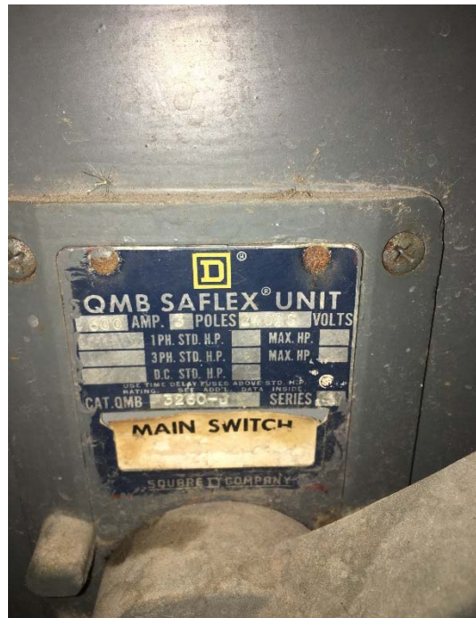
Photo E5 Corroded main breaker
