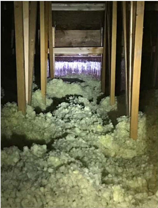
Photo Client3 View of attic space with daylight and significant ice buildup visible.
