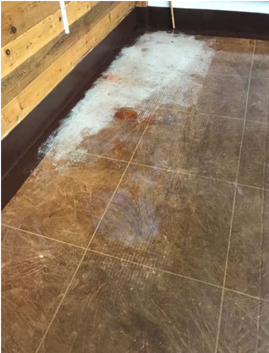
Photo Client5 View of frost buildup on floor in the original fitness room.
