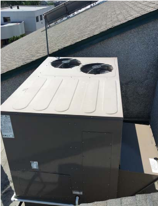
Photo M3 Fitness Area (RTU)
