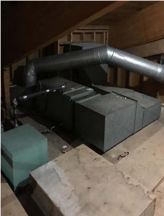
Photo M5 Meeting Room (AHU)
