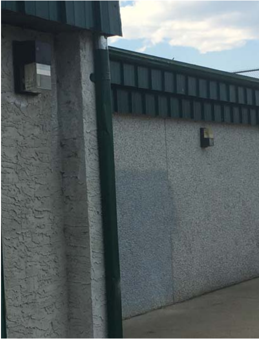
Photo E7 Exterior Lighting
