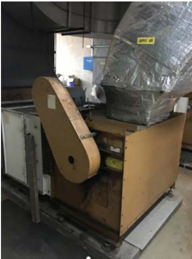
Photo M1A Pool Lobby (AHU)
