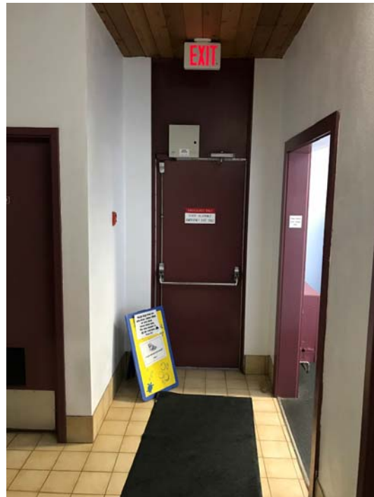
Photo A20 Interior view of exit door at West side of fitness room.
