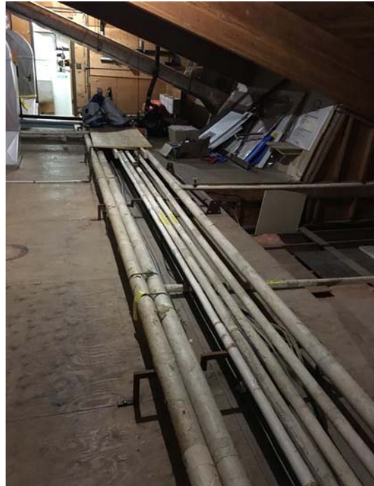
Photo M6 Plumbing Piping Attic
