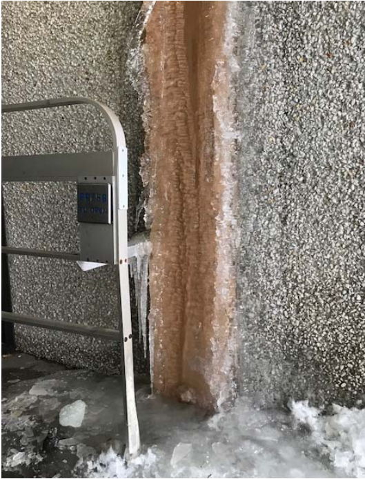
Photo Client1 View of ice buildup at structural column on South side the main entrance
