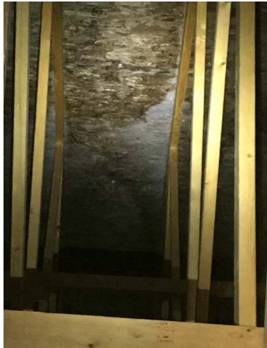
Photo Client4 Underside of roof sheathing with significant signs of moisture and frost.
