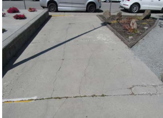
Photo S8 Cracks on concrete paving at front entrance.
