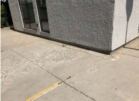
Photo S7 Spalling and differential settling of pavement at main entrance creating a tripping hazard.
