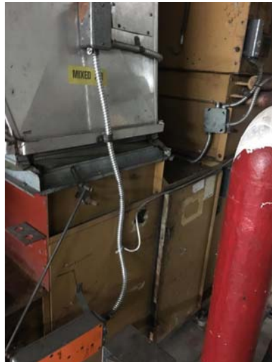
Photo M1B Pool Area (AHU)
