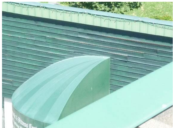
Photo Env5 Wood Cladding and entrance canopy creating snow trap.
