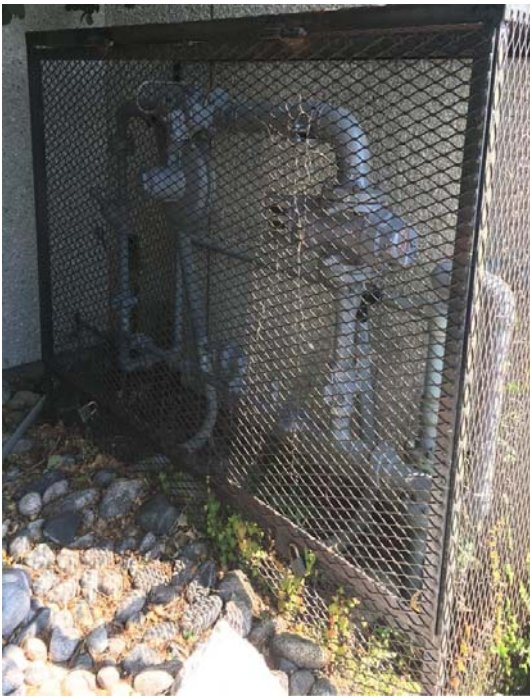
Photo M11 Gas Meter Enclosure
