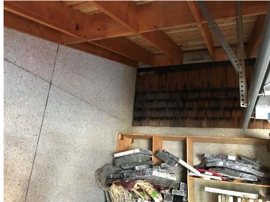
Photo A8 View inside storage area looking toward exterior wall of original facility.
