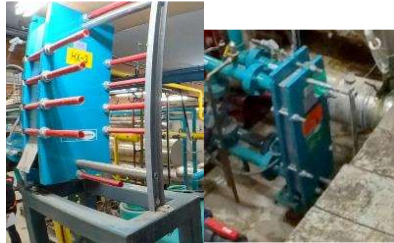
Photo #M16: Heat exchangers.
