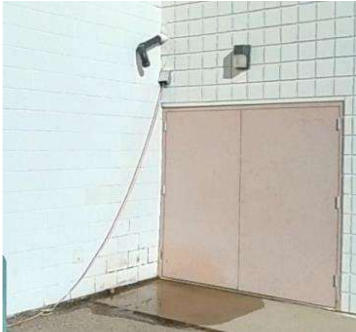
Photo #M25: Drainage issue at SW building corner.
