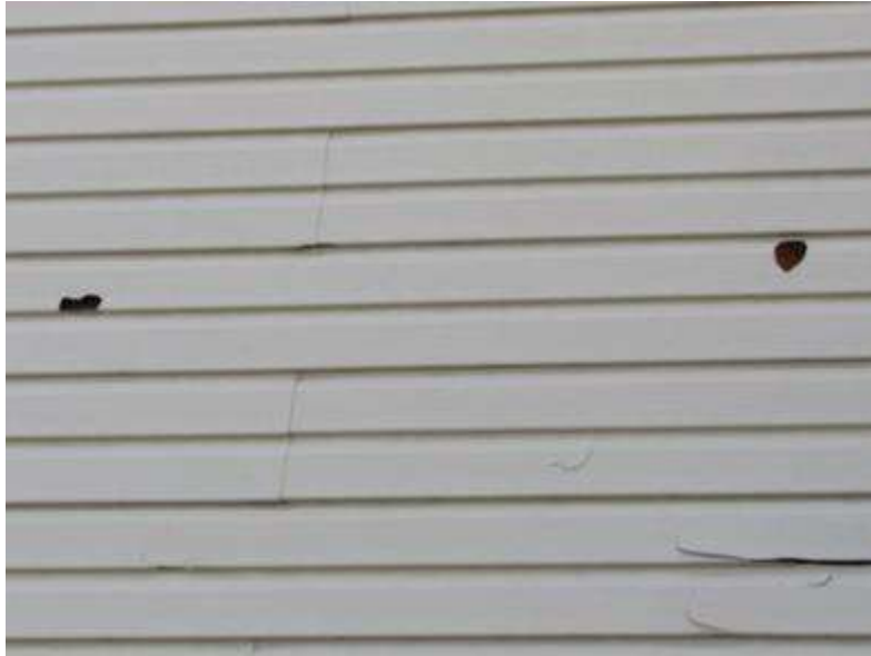
Photo #A5: Damages of vinyl siding.
