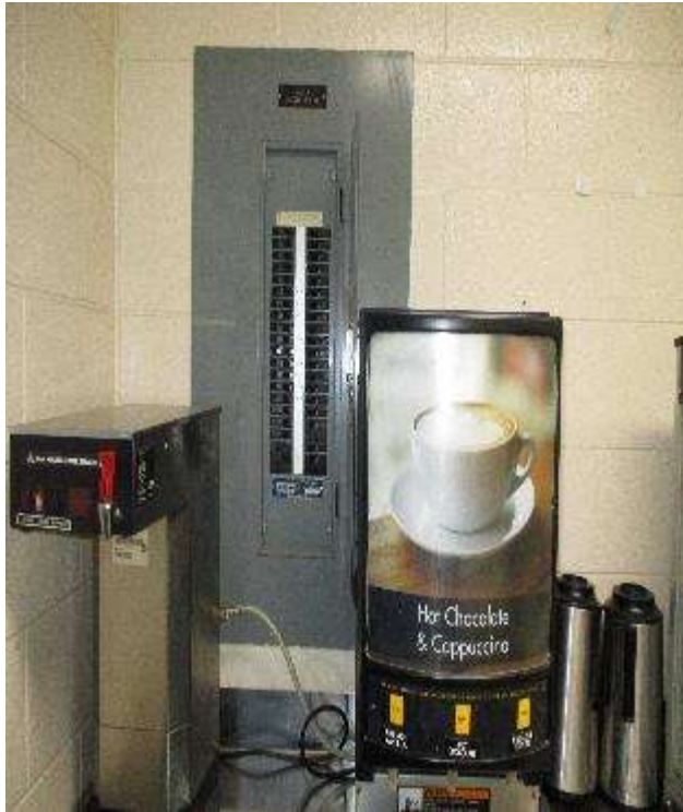
Photo #E7: Subpanels in Concession Area 120/208V.
