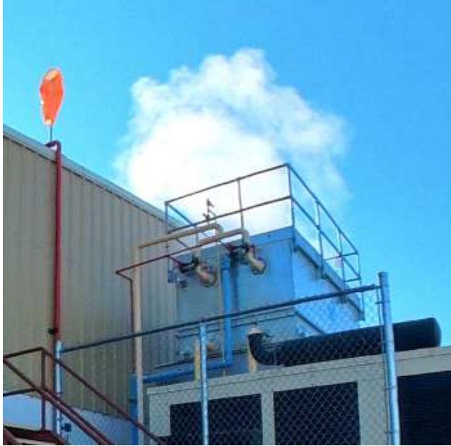
Photo #M35: Excessive heat rejection through Evaporative Condenser.
