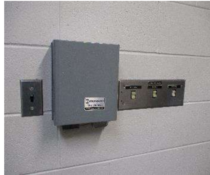
Photo #E14: Typical curling rink lighting control timer and switch bank
