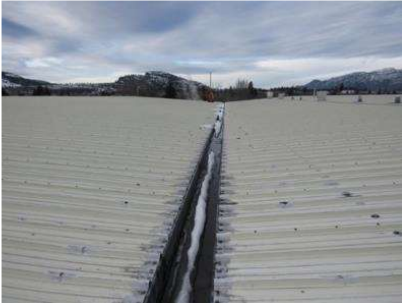
Photo #A23: Sloped metal roof. An active water leak was observed around the metal trench gutter. Localized repair areas also observed.
