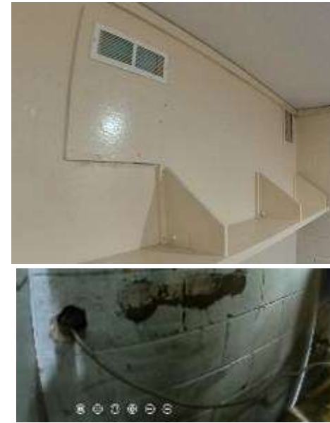
Photo #M32: All Grilles are blocked off at Room #6. Numerous locations where fire sealant missing.
