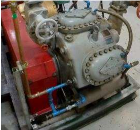
Photo #M15: Compressor (Typical).
