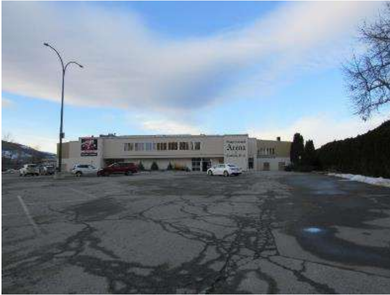
Photo #A1: Longitudinal and alligator cracks caused by freeze thaw and age of surface in the parking lot area.
