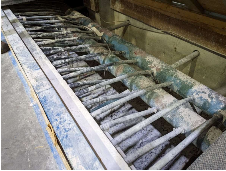
Photo #S5: Steel header pipes (Corrosion observed).
