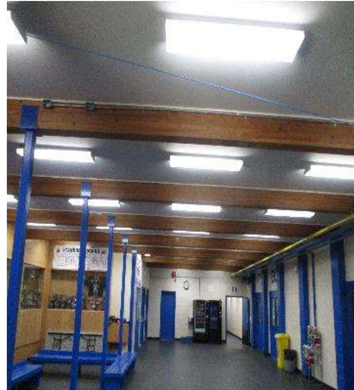
Photo #E10: Typical fluorescent strip lights in Lobby.
