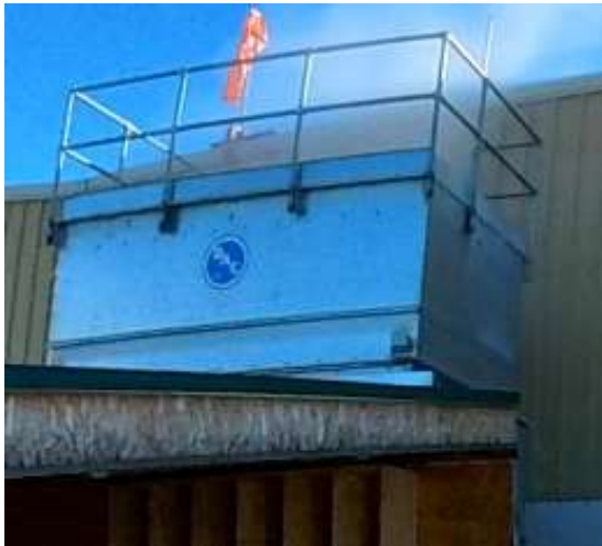
Photo #M13: Evaporative Condenser.
