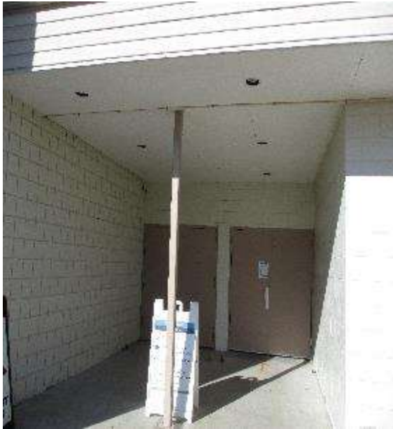
Photo #E15: Typical soffit mounted exterior lighting in the building- wall mounted units similar.
