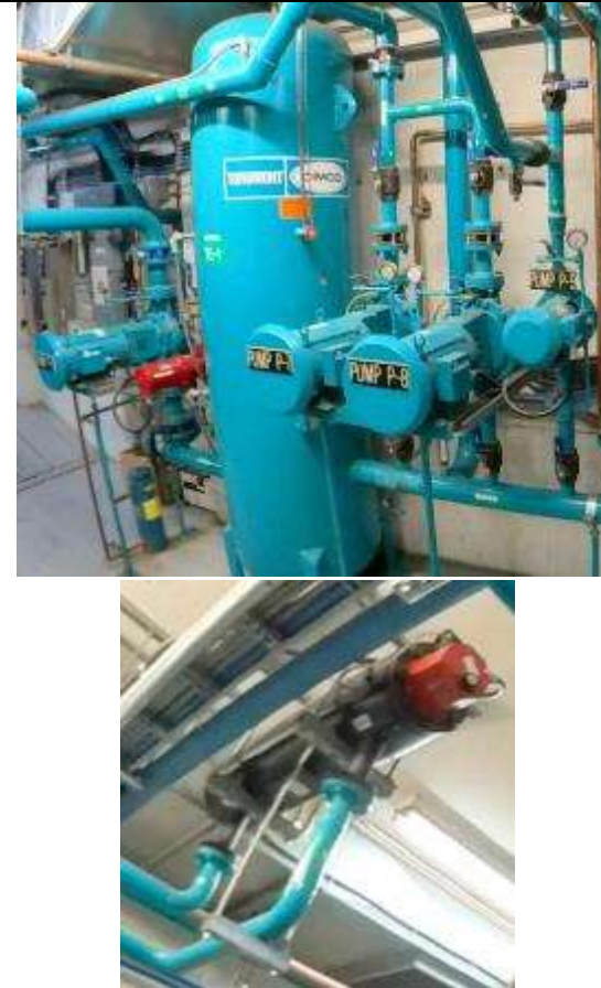
Photo #M8: Thermal Equalizer with Water Pumps and back-up Water Electric Heater.
