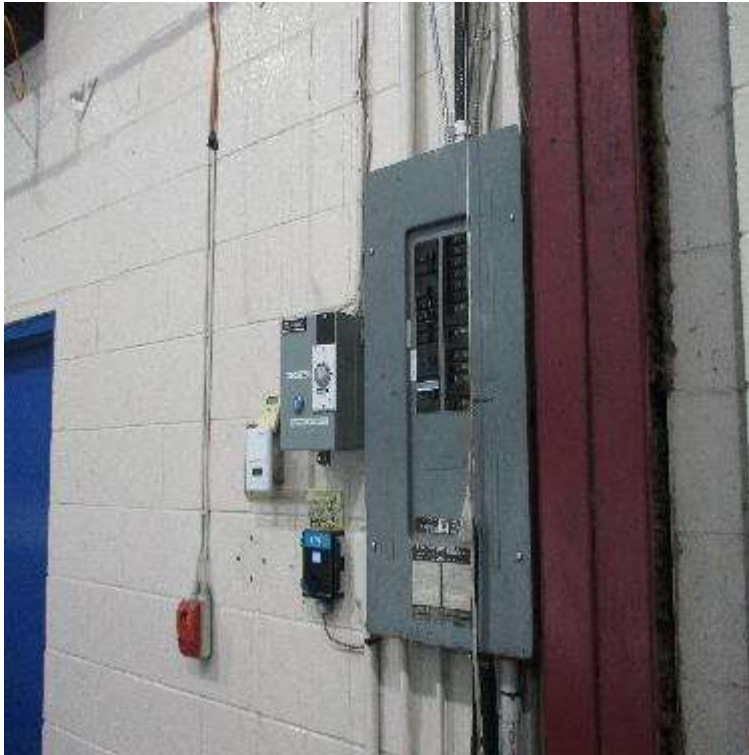
Photo #E3: Sub distribution Main Panel board - 200Y/120V located outside of maintenance room.
