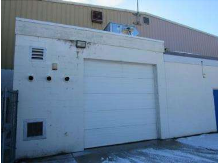
Photo #A7: Typical overhead door.
