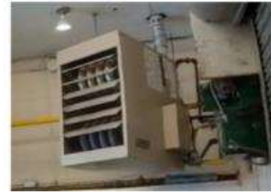
Photo #M4: Typical Gas-Fired and Electrical Unit Heaters (Typical).
