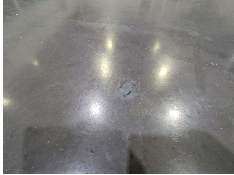
Photo #S6: Evidence of localized repair on SOG.
