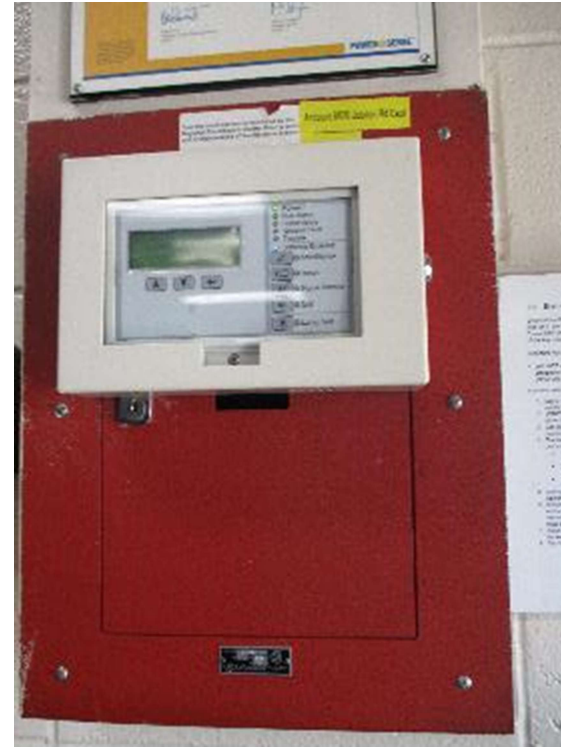
Photo #E4: Fire Alarm Annunciator at main entrance.
