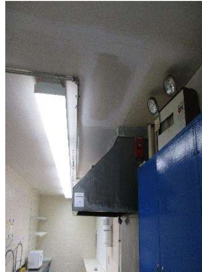
Photo #E6: Concession Area Surface mounted Fluorescent recessed lighting and Legacy emergency battery pack with heads
