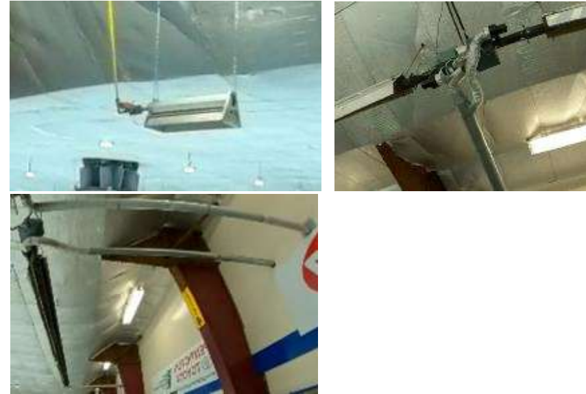
Photo #M12: Infrared heaters in Ice Rink area (Typical).
