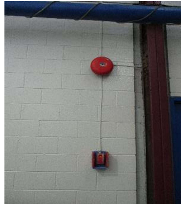
Photo #E12: Typical fire alarm pull station and bell in the building.
