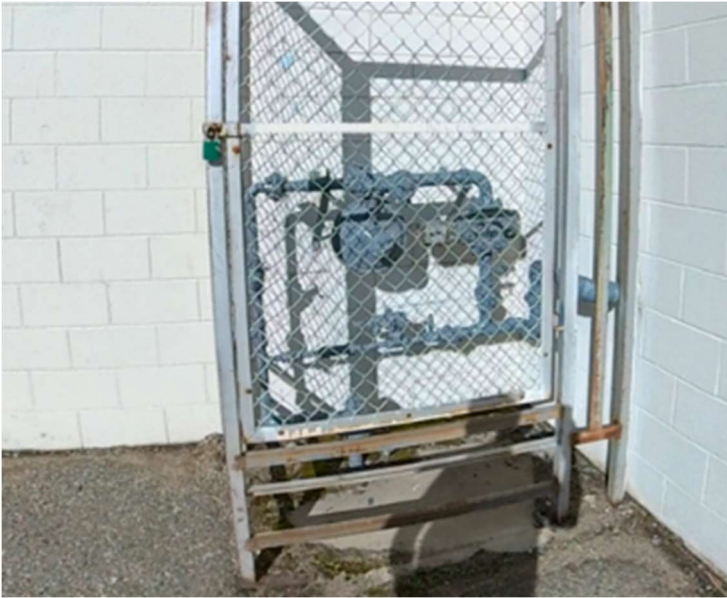
Photo #M1: Gas Meter at SW building corner.
