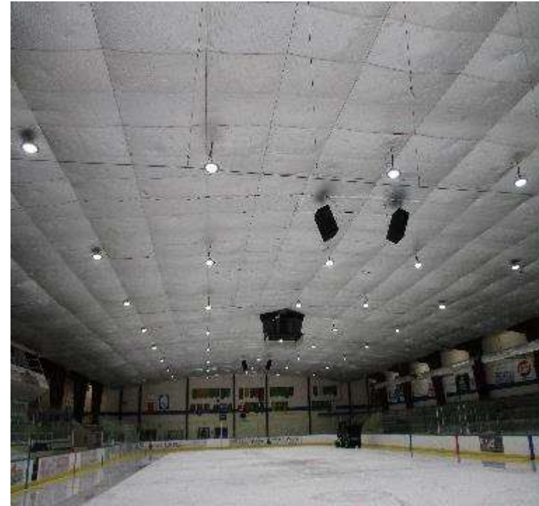
Photo #E8: Suspended LED lights located in the Ice Arena Rink.
