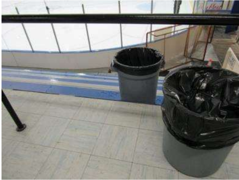
Photo #A13: 2 nd floor of Ice arena. Buckets were observed in the water leak area.
