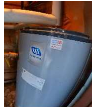
Photo #M6: Hot Water Storage Tanks.
