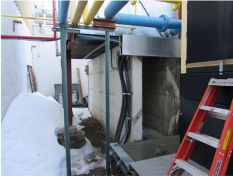
Photo #S11: Metal and CIP structures for the mechanical equipment.
