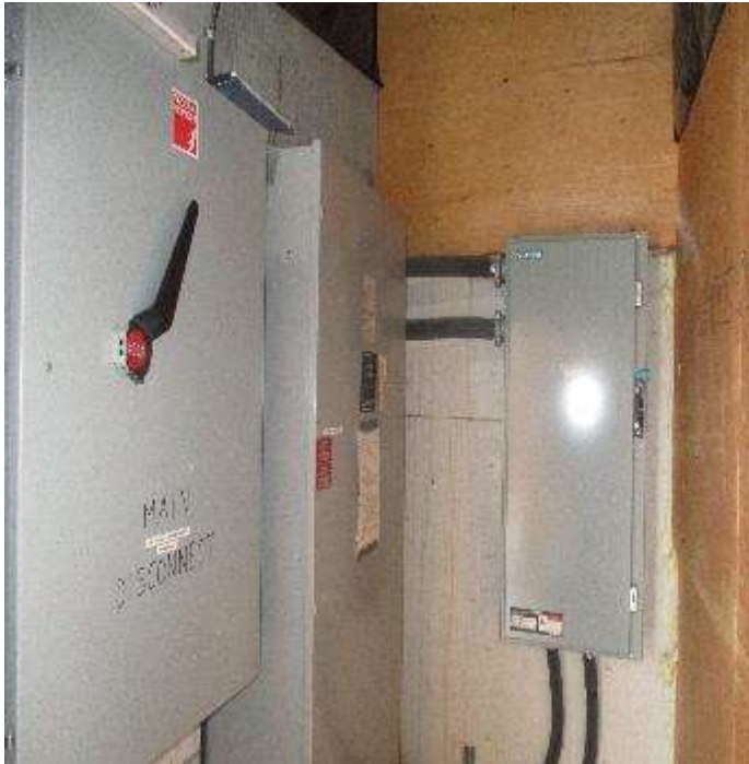
Photo #E17: Emergency distribution, transfer switch and panel.
