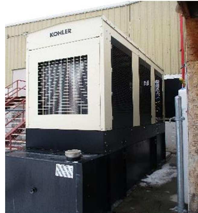
Photo #E18: Packaged Exterior Generator.
