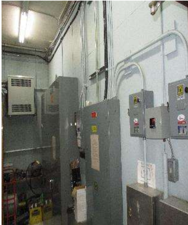
Photo #E1: Mai Electrical Room. (Transformer, switchboard, panels and disconnect.)
