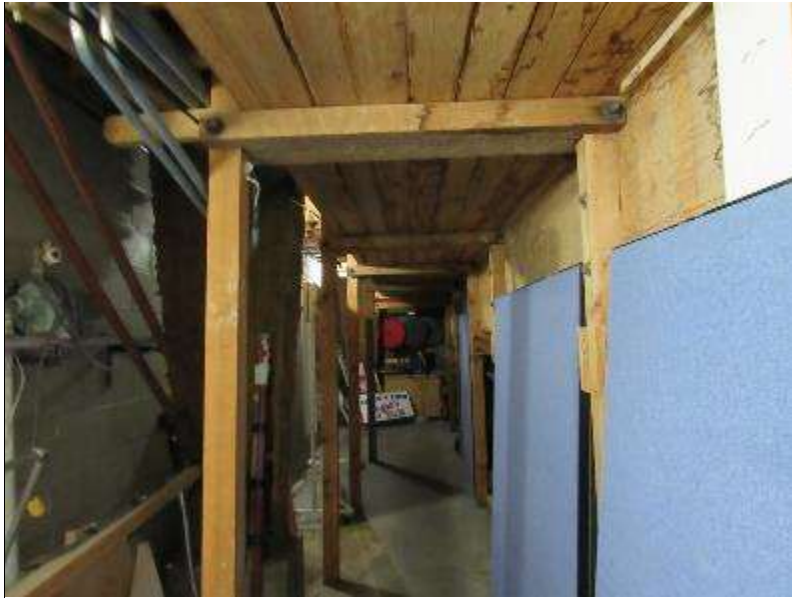
Photo #S9: Exposed framing in storage room under bleacher areas.
