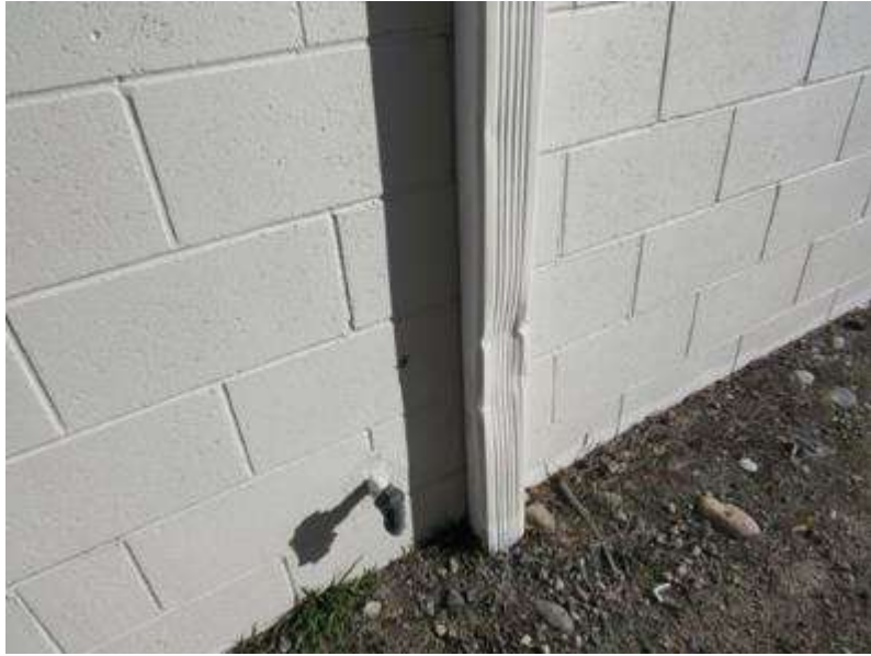
Photo #A25: Dented metal downspout.
