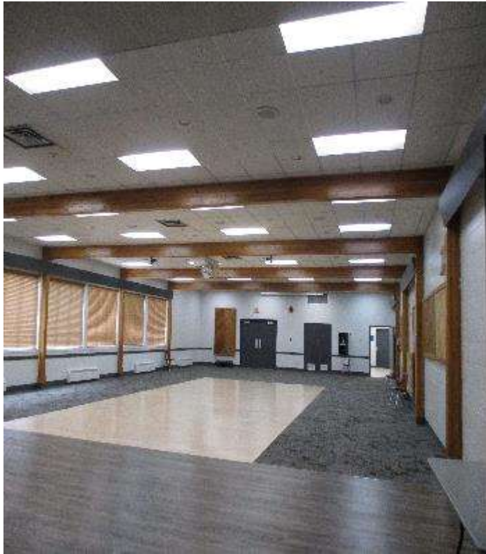
Photo #E9: Typical Events area LED recessed lighting and Pot Lights
