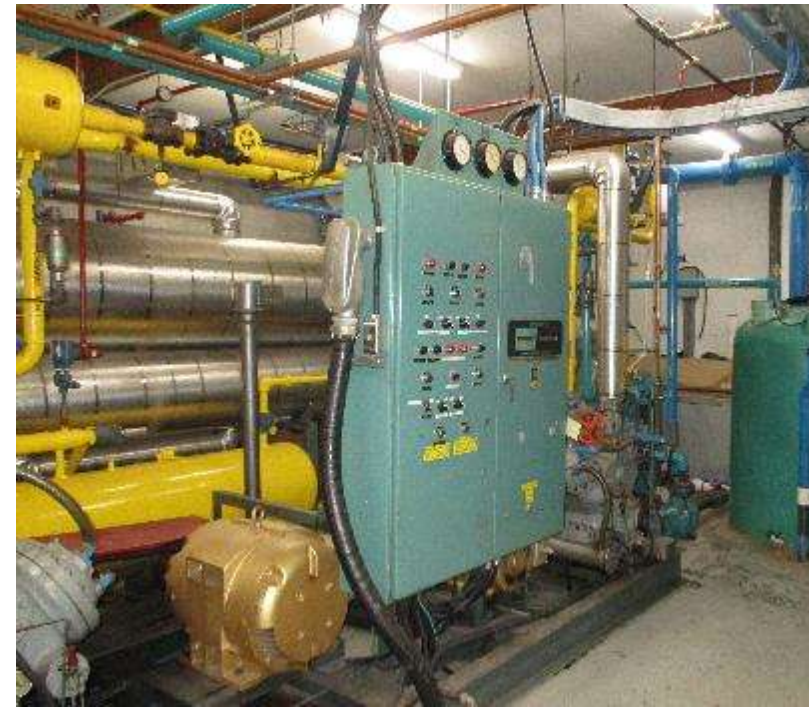
Photo #E2: Ice Plant Control Panel.
