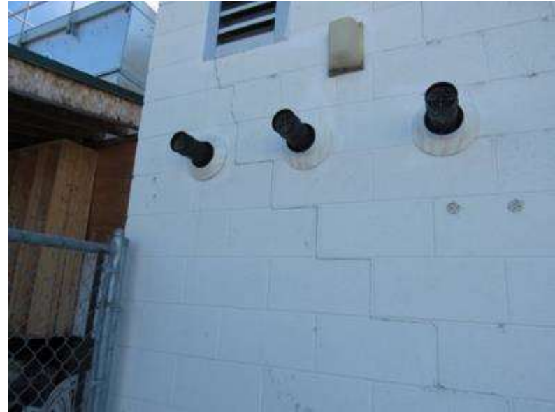
Photo #A6: Step crack on the concrete block wall.
