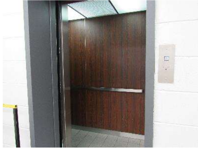
Photo #A26: Elevator cabin.
