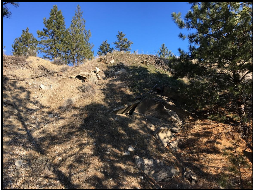
Photo 12: A view of buried concrete on-site located in the central storage area along the north boundary.
