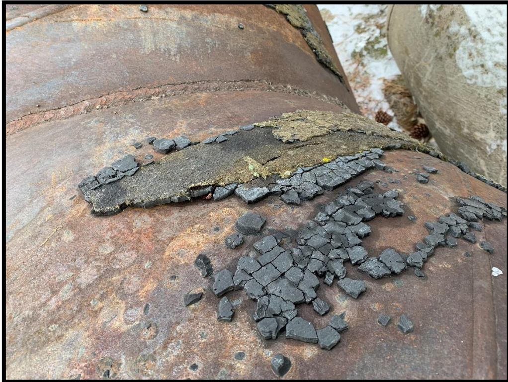
Photo 6: A closeup of the material on the pipes that is potentially ACM wrap.
