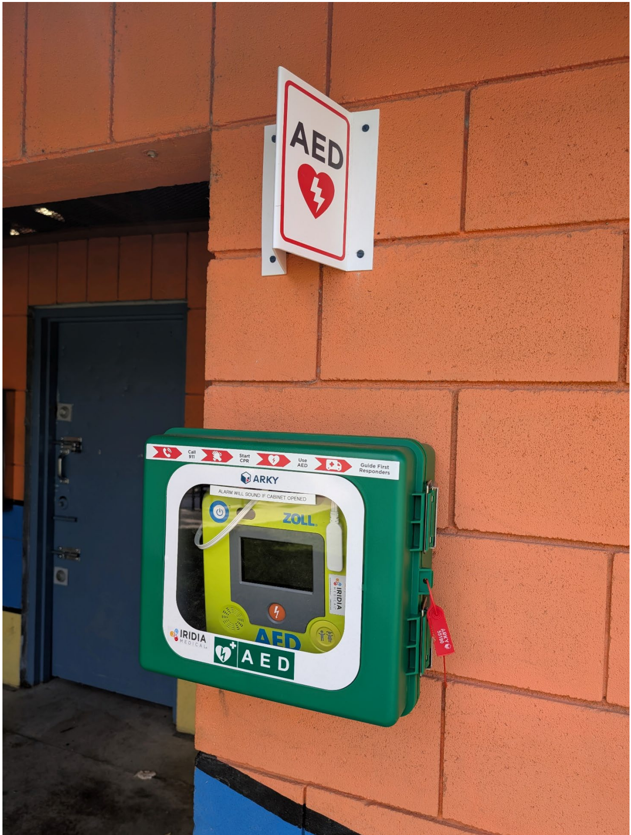
Photo 7 – New AED on the exterior of the Peach Orchard Beach Washroom Building
