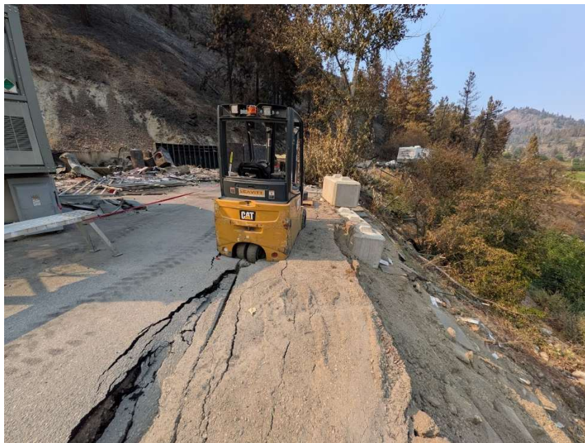
Photo 6. Failed retaining wall on 16218 Garnet Valley Rd.
