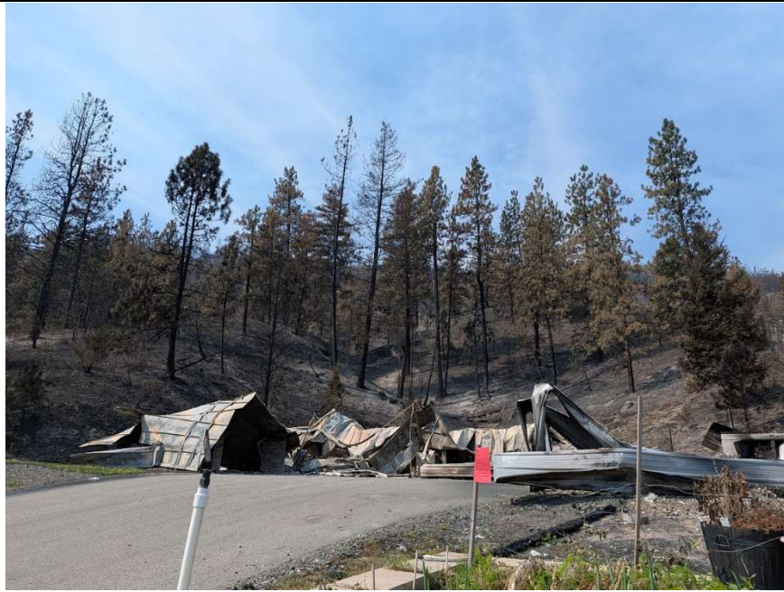
Photo 3. Burned gully with previous building immediately at the base.
