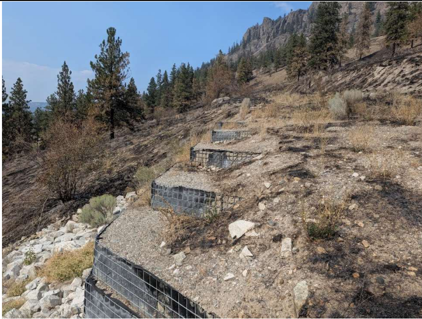
Photo 11. Damaged gabion wall upslope of 21207 Garnet Valley Rd looking north.
