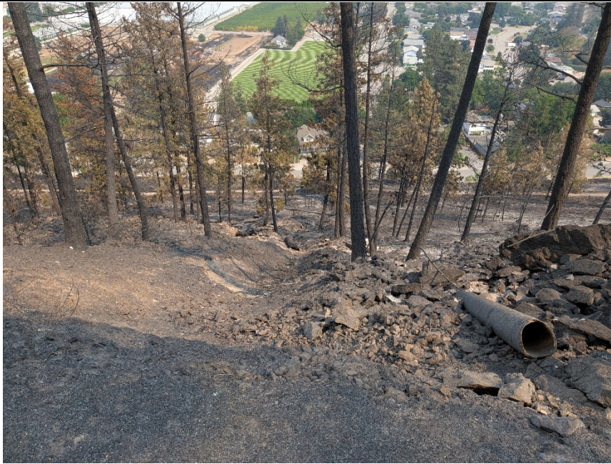
Photo 5. Slope uphill (west) of Cartwright Ave looking east, at pre-existing erosion channels.
