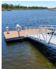
Floating dock and ramp
