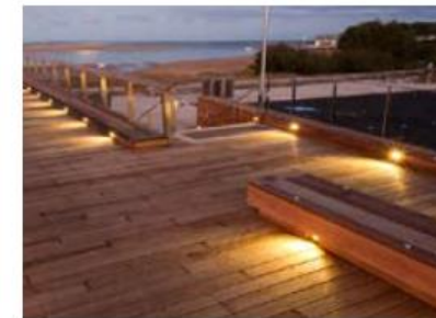
Electrical distribution (no fixtures)
