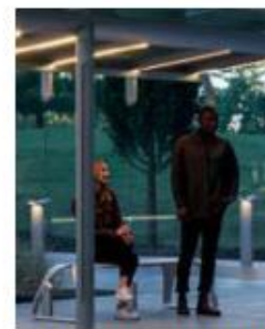
Solar lighting fixtures in shade structure
