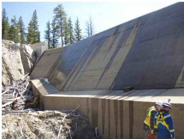
Photo 3 Spillway Gallery - Air Intake
