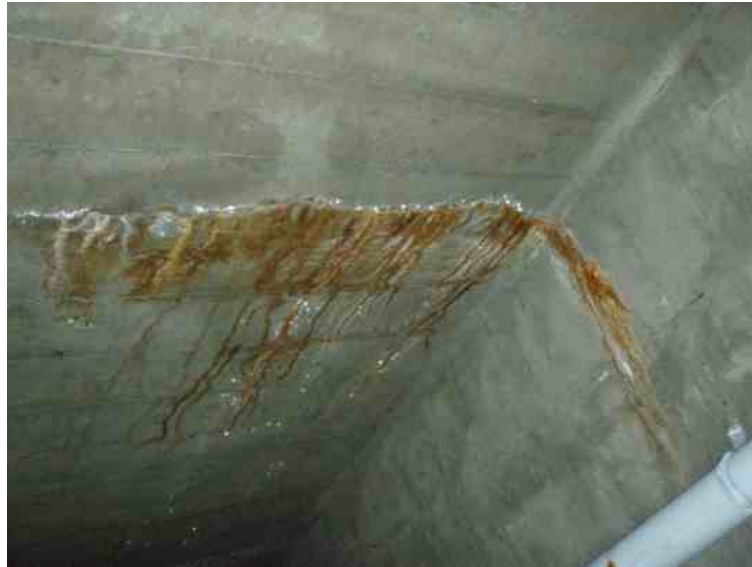
Photo 6 Block 12 – Weep on Upstream Face
